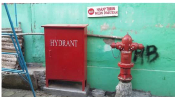
Fig. 2. Hydrant installation – an existing example of government intervention to disaster mitigation at kampung Ngampilan.
