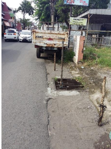
Fig. 4. The narrow and inaccessible pathway, the parked vehicle and vulnerable gratings causing access difficulty for pedestrians.
