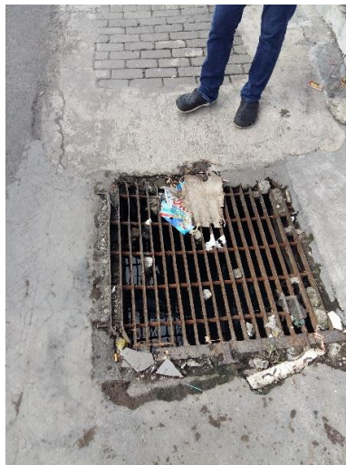
Fig. 5. The vulnerable gratings as one of the obstacles that pedestrians faced at the sidewalks.
