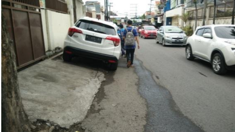
Fig. 7. The sidewalk which cross slopes exceeded 1:50 causing more danger for pedestrians who were using crutch, walking stick or wheelchair.
