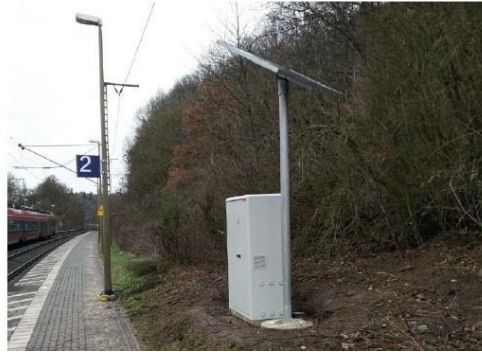
Fig. 11. Stationary installation in Friedhausen (next to Giessen).
