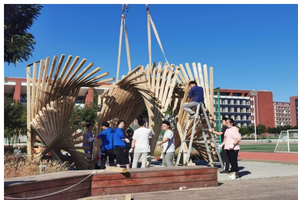
Fig. 2. 2020 Beijing Robot Arm Digital Construction International Work Camp - Robot Arm Work Camp Wooden Structure Construction Process
